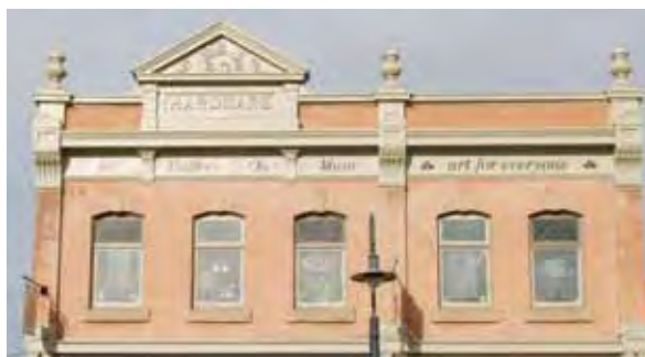
The two remaining decorative sheet metal urns at the top of the façade of the M & J Hardware Building in Lacombe, AB were determined to be beyond repair due to weathering over time. A third sheet metal urn (centre) was missing. The existing deteriorated elements and photographic documentation were used to replicate these elements. The M & J Hardware Building is an example where missing features from the restoration period have been re-instated based on physical and documentary evidence.
