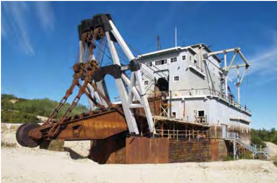
The deteriorated heavy timber bow gantry frame of Dredge No. 4, in Dawson City, YK, was dismantled and replaced in kind with a new frame, built from new timbers sized to match the original timbers and reusing all original metal brackets and fixtures. The bow gantry, which supports the digging ladder, is a significant constructed element in the dredge's operational design.
