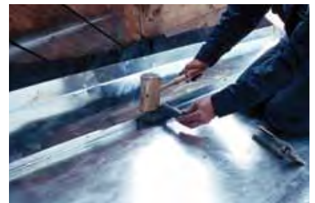
When restoring the former post office in Dawson, YK, the metal roofing surface, which was too deteriorated to repair, was replaced in kind. Physical evidence from the restoration period was used as a model to reproduce the characteristic standing seam detail.
