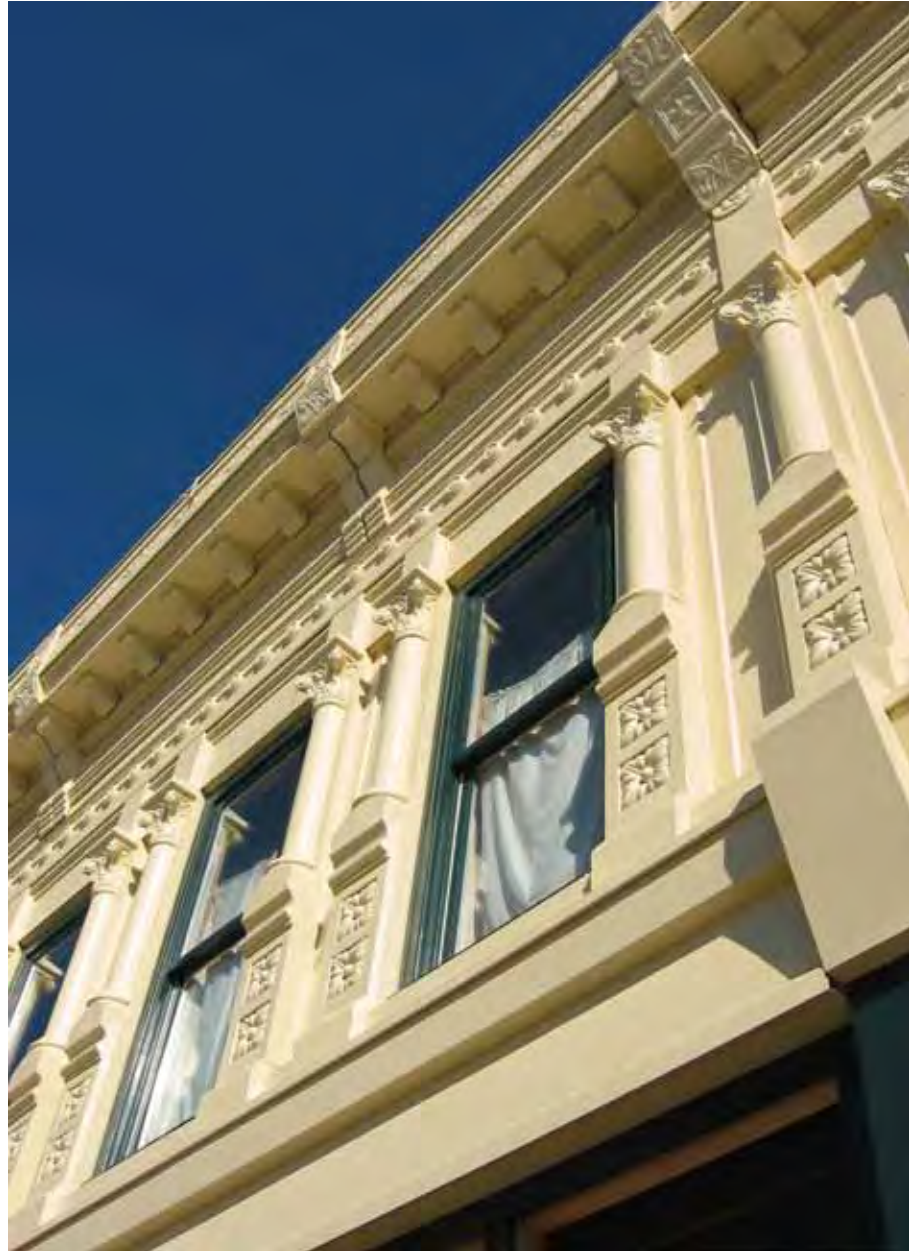
Detail of pressed metal facade after rehabilitation, showing the hallmarks of the original Mesker design. The work consisted of the following: removal of the metal panels, carefully identifying their original locations; removal of multiple layers of paint using a chemical bath; recoating with an epoxy-based paint system; and reinstallation in the original locations on furring strips according to a rain screen principle.
