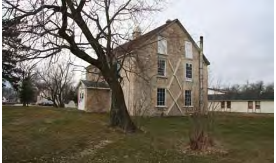
It is important to adapt interim stabilization interventions to the anticipated lifespan of the intervention and make it as reversible as possible. Temporary steel cross bracing supports an exterior wall at St. Peter's Dynevor Anglican Church Rectory in Selkirk MB.
