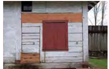
A condition assessment of the exterior walls and frame of this Storehouse at Fort Langley, BC found extensive deterioration of some timbers, which required replacement in kind. The dimensions, hewn finish and species of wood used in the repairs matched those replaced. The photograph shows part of one storehouse wall after the repairs were completed, but before the new timbers were whitewashed.
