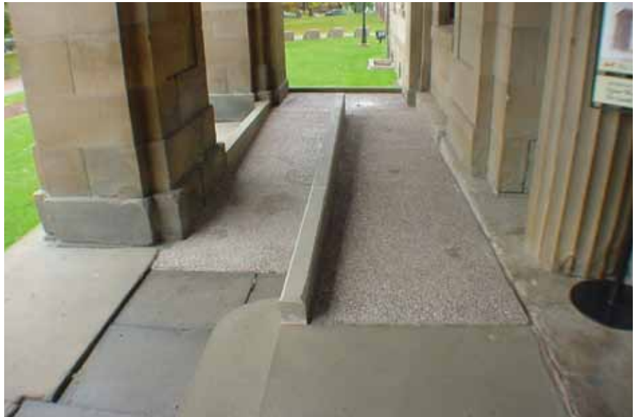
Adding a ramp to meet accessibility requirements should be designed to be compatible with a building's character. This new ramp at Province House in Charlottetown was discretely integrated into one side of an existing entrance porch.
