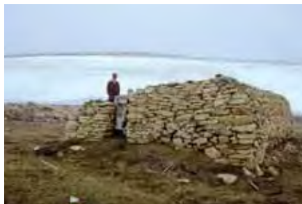
Responding to the dangers of arctic exploration and the loss of the Franklin Expedition, Kellett's Storehouse in Nunavut was built in 1853 for sailors in distress. Constructed from local stone, it was filled with enough provisions to maintain a large group for several months. Conserving building remains or above-ground archaeological resources pose unique challenges. In this case, the walls and foundations were stabilized and an insulated floor was installed allowing remaining soil layers and associated artifacts to be left in place while being protected from theft and further exposure to the elements.
