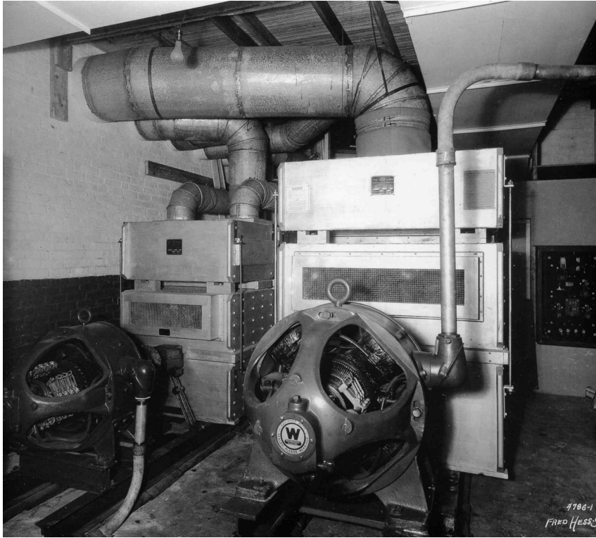
Figure 13. Two of Atlantic City's Electrical Wind Blowers
