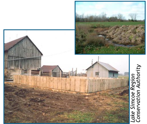
Portage Road Farm Upgrades – uncovered manure pile (top right) and the construction of a new manure storage facility to minimize non-point source runoff into local streams.
